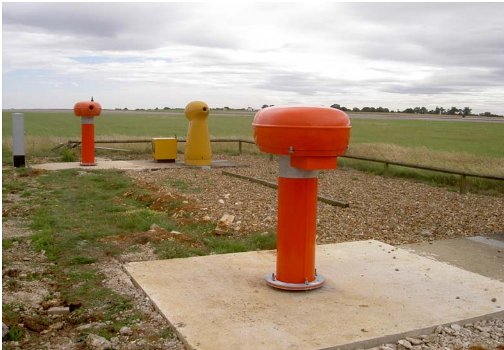
Figure 1 Field Site Installation
